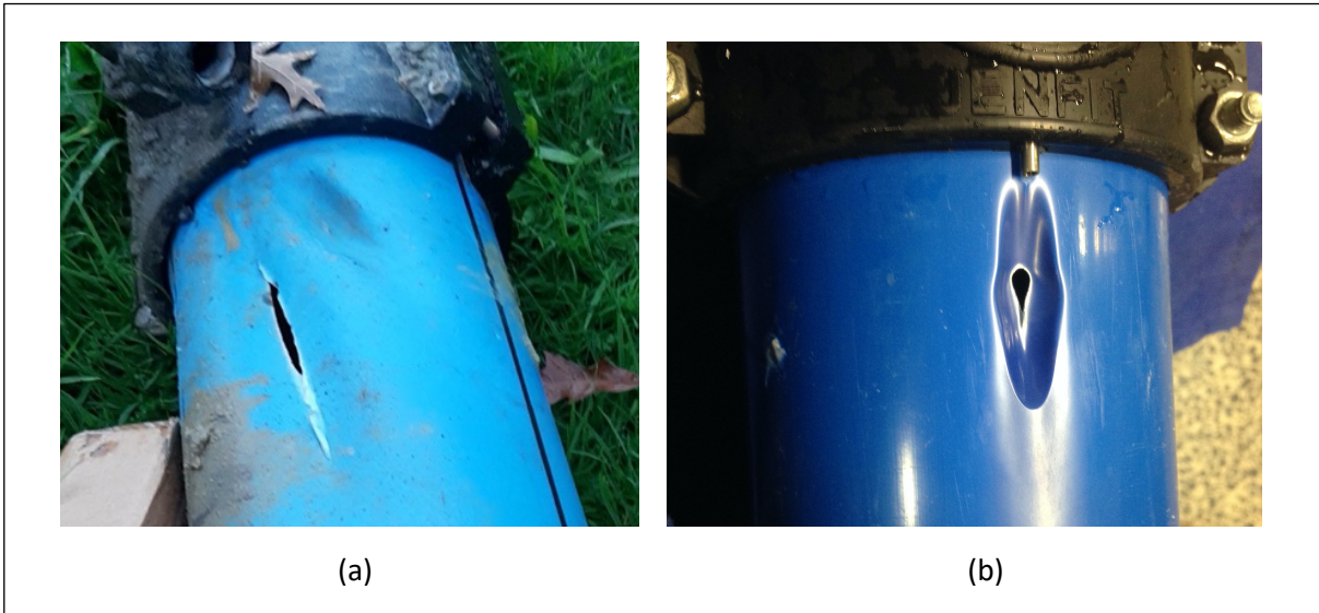
Figure 4 a) A failed 180 mm diameter PE pipe caused by soil erosion driven by a water jet from a leaking collar and b) a similar failure from a laboratory study (Pike, 2018)
