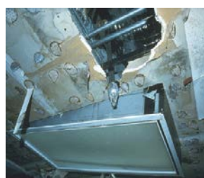
a. Fractured elbow joint
