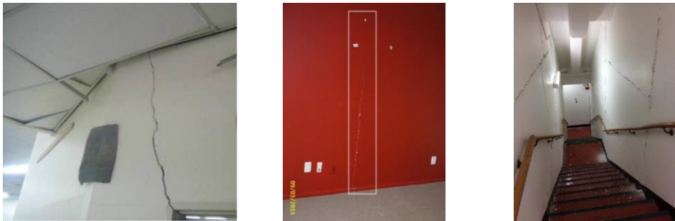
Fig. 7 – Damaged partition walls [3,13,40]
