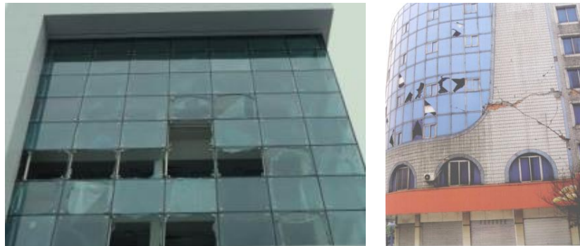
Fig. 11 – Glazed Curtain Wall Damages [4,43]
