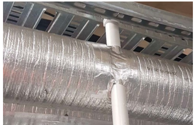
Figure 5: Clash of pipe with insulated pipe and cable tray
