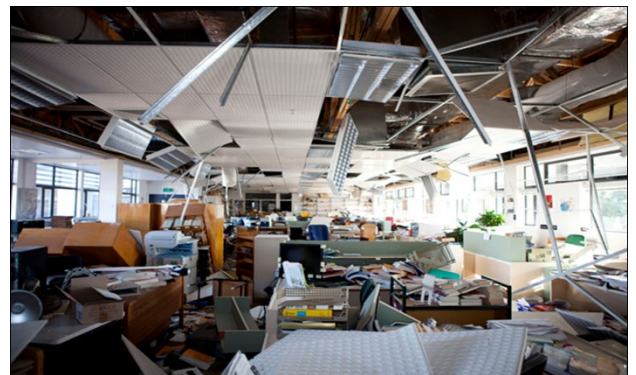
Figure 1: Illustrating damage to non-structural elements observed in the Canterbury earthquakes (from Dhakal, 2010)
