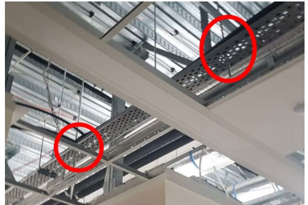
Figure 4: Ceiling hangers run through cable tray
